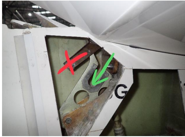
Disconnected elevator control
